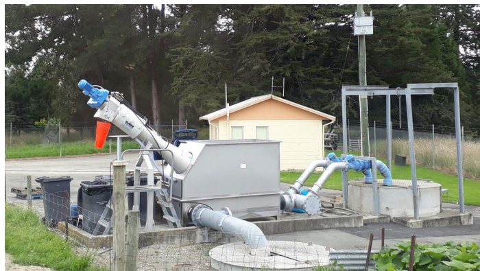
New milliscreen for the waste water treatment plant
