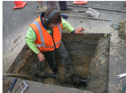
Water Supply - Urban
