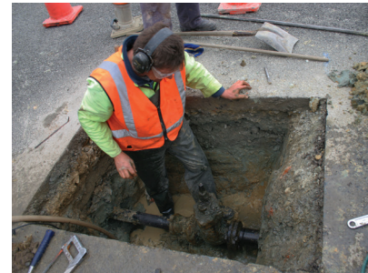
Water Supply - Urban
