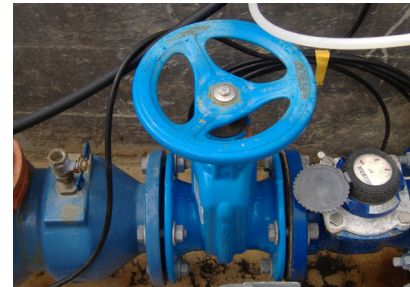
Water Supply - Urban
