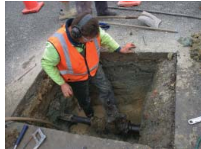
Water Supply - Urban
